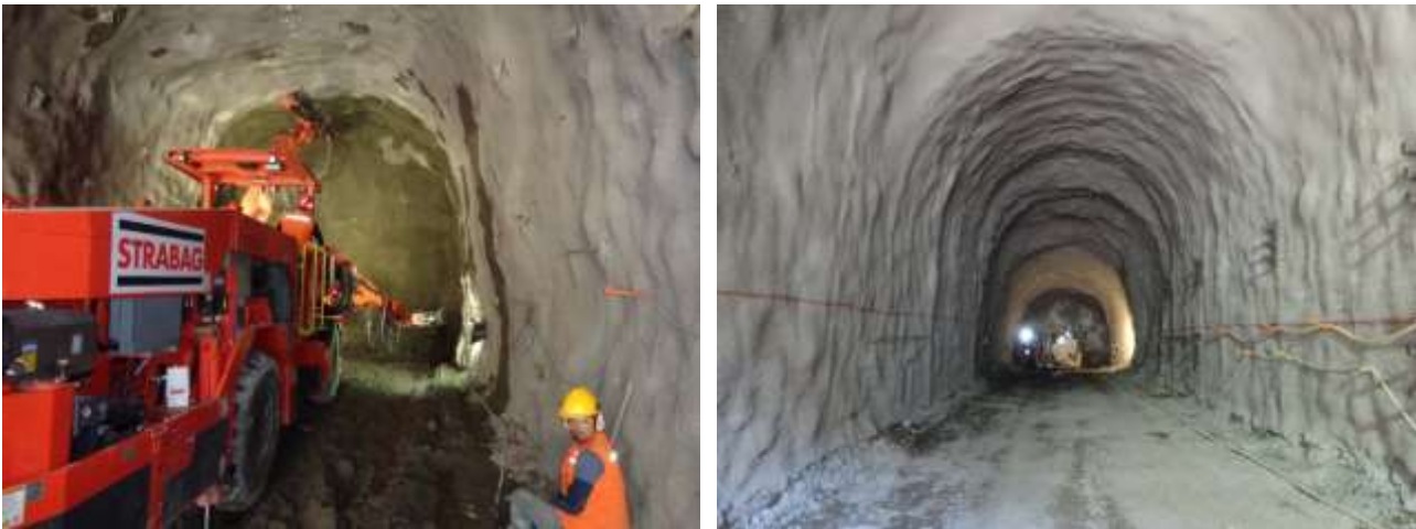
Figure 9.: Conventional tunnel excavation by blasting at the beginning of tunnel VI, application of a machine (boomer) with 3 arms for drilling holes for blasting and for laying anchors (left) and a view of the beginning of tunnel excavation VI with primary support by sprayed concrete and anchors.
