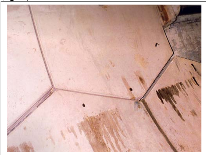
Figure 12. Imperfections in radial and longitudinal joints.
