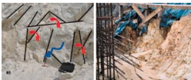
Figure 3- a) Discontinuity controlled block / wedge failure in jointed granitic rock mass, b) Erosional / piping failure in disintegrated soil-like granitic rock mass.
