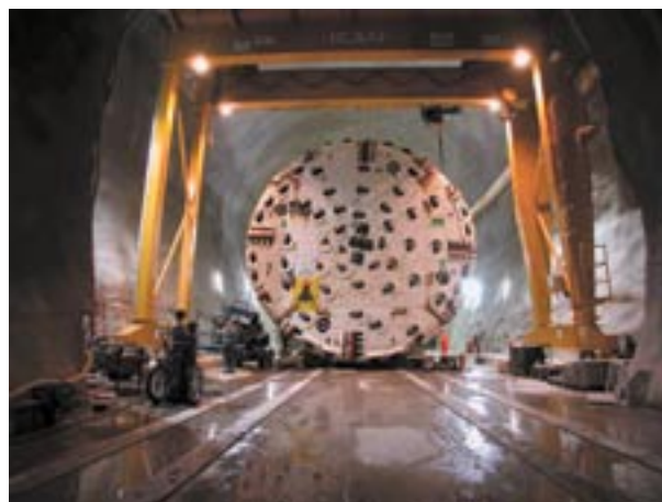
Fig. 16: Tunnel Bodio, unexpected fault zone "Tm 2,705".
