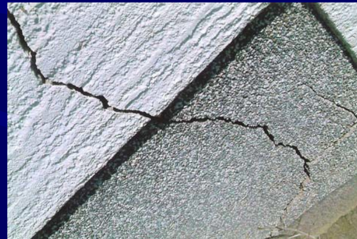
Cracks in buildings on faults
